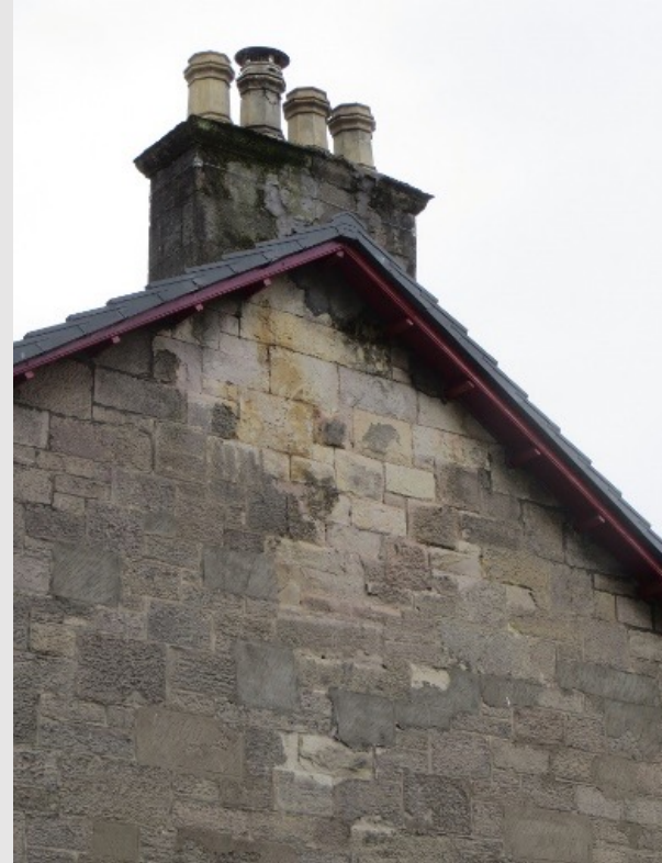
Stone erosion and chimney defects
