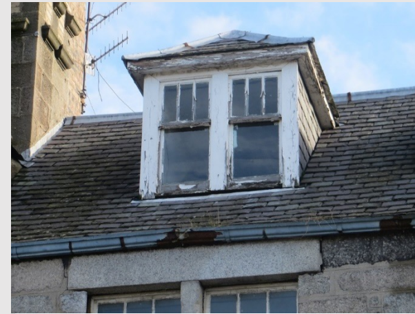
Lack of regular repainting of dormer window joinery
