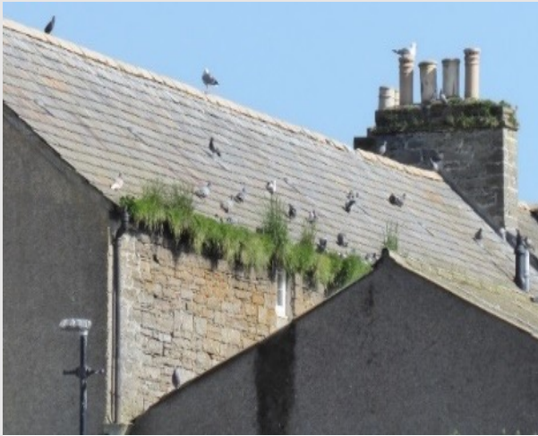
Lack of gutter clearing
