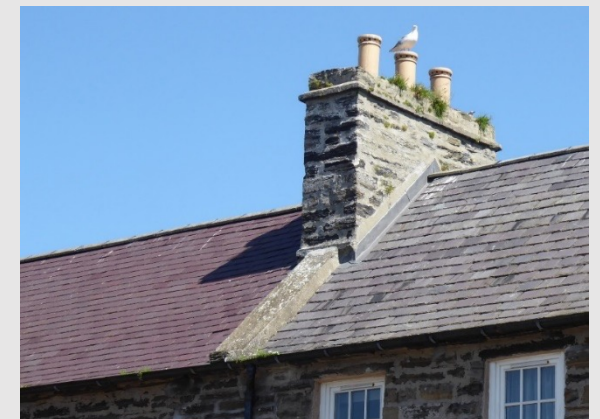
Inappropriate slate specification
