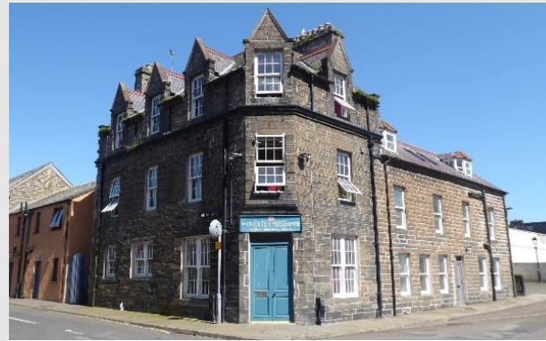
Loss of original windows and inappropriate replacements
