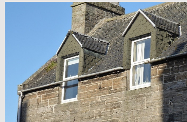
Inappropriate felt tiles used on dormers
