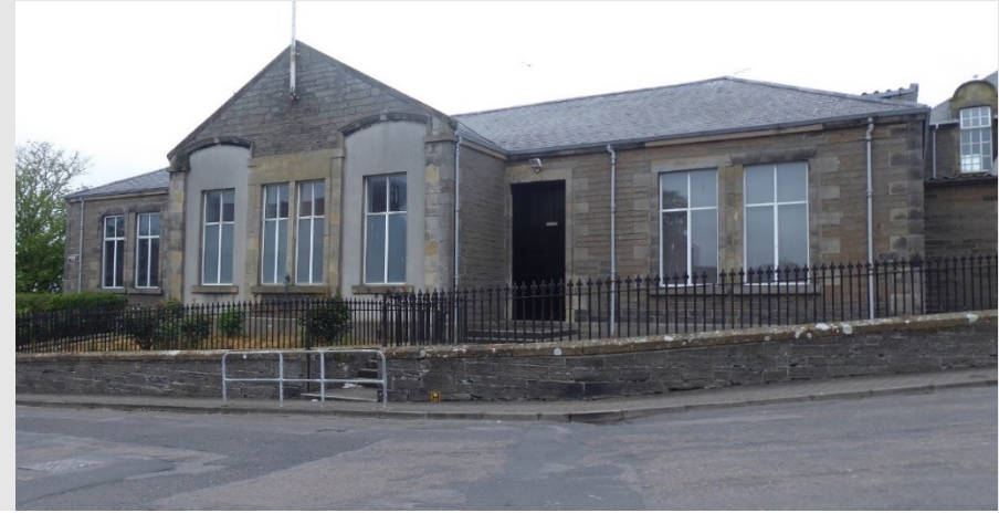
Building stripped of its architectural features has removed much of the building's original character.
