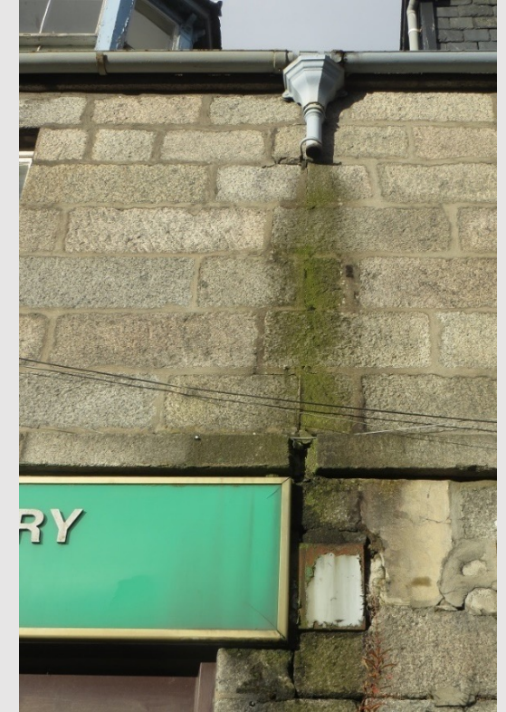
Missing rainwater goods
