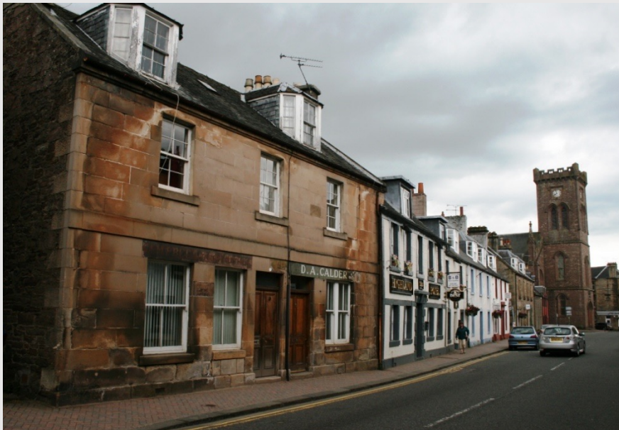
Historic buildings effected by disrepair
